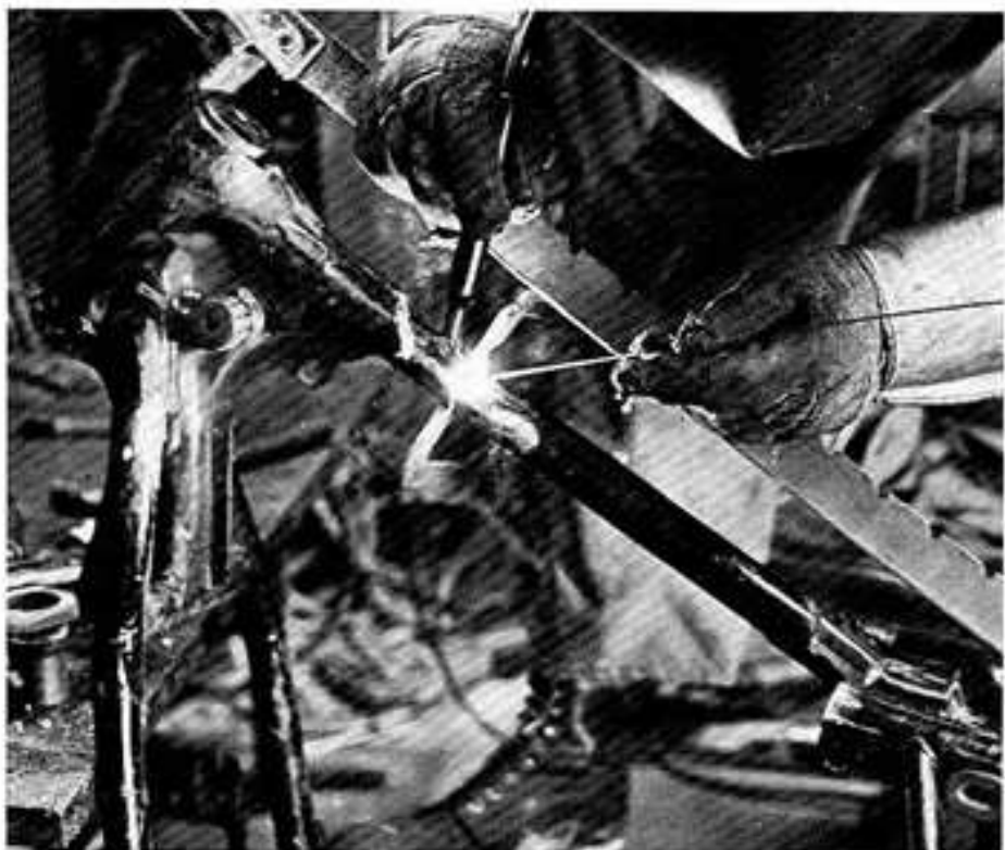
Close gap with large clamp and have frame heli-arc'd by an expert welder.
